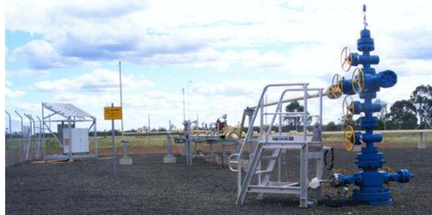
^Compression facility Silver Springs UGS
